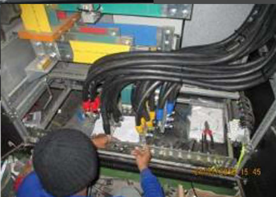
Automatic Transfer Switch (ATS) Implementation
