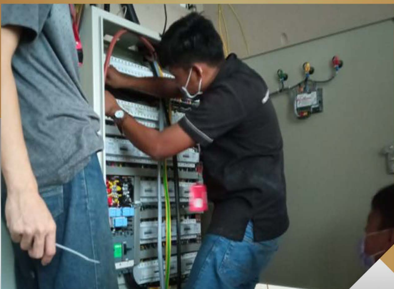
DC Main Distribution Panel Implementation
