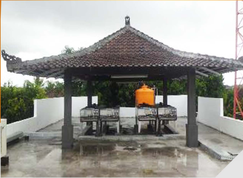
Rooftop : Outdoor PAC, AC Split, CCTV Camera & Bale Bengong as cover outdoor PAC
