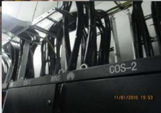
Change Over Switch (COS) Implementation
