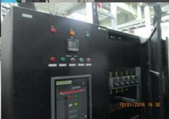
DC Main Distribution Panel Implementation
