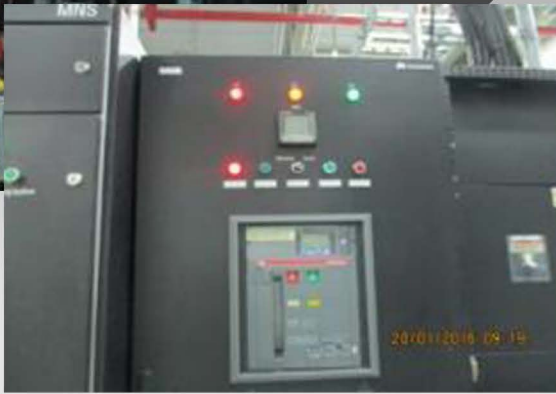
Utility Main Distribution Panel Implementation
