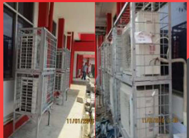
Outdoor Condensor Installation
