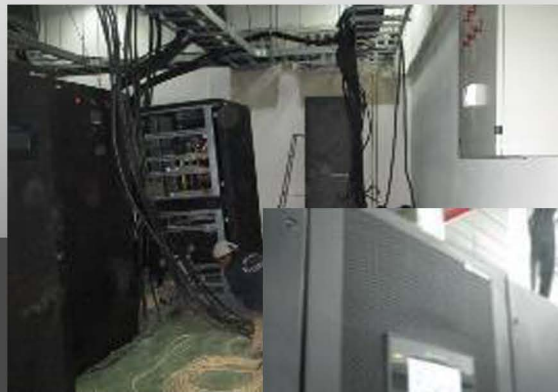
Uninterruptible Power Supply (UPS) Implementation
