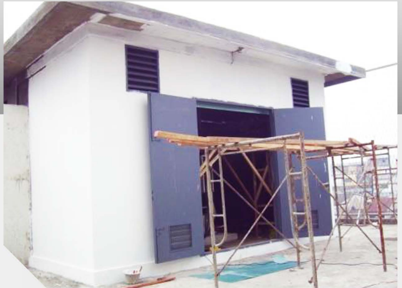
Power / Genset house
