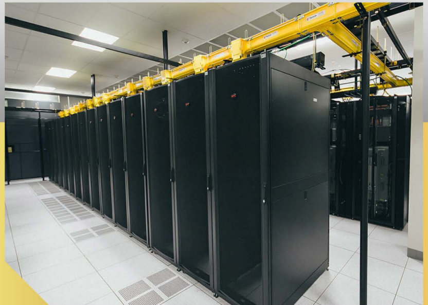
Data Center Huawei, Jakarta
