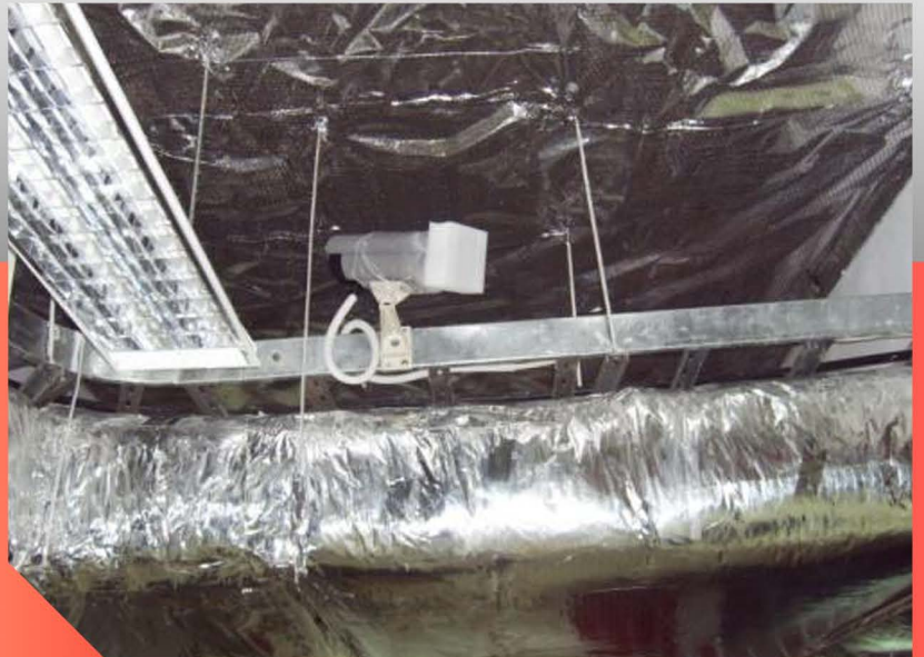
Air Con, Lighting, Cabling & CCTV
