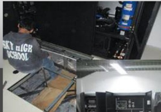
Precision Air Conditioner (PAC) Implementation
