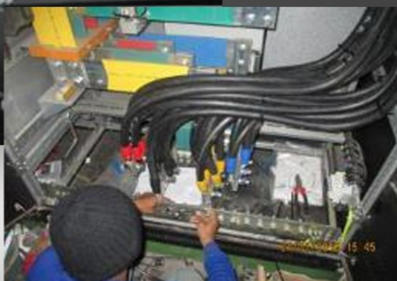
Automatic Transfer Switch (ATS) Implementation
