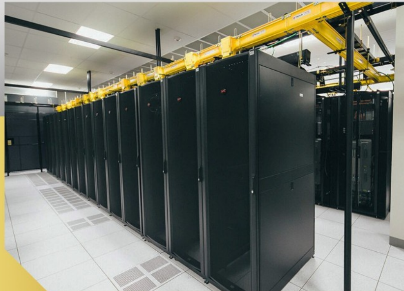
Data Center Huawei, Jakarta
