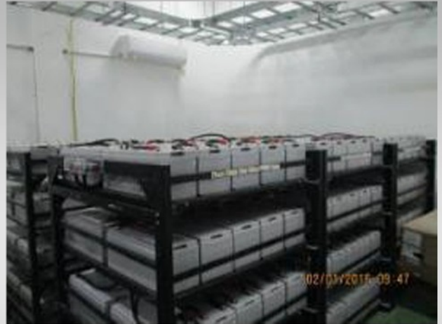
Battery & Racks Installation
