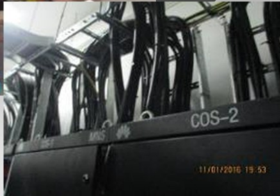
Change Over Switch (COS) Implementation
