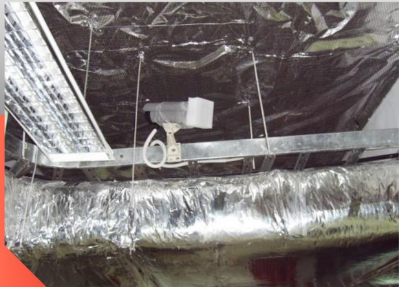
Air Con, Lighting, Cabling & CCTV
