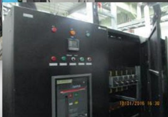
DC Main Distribution Panel Implementation
