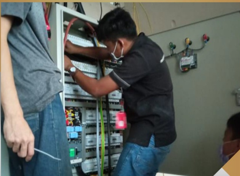
DC Main Distribution Panel Implementation
