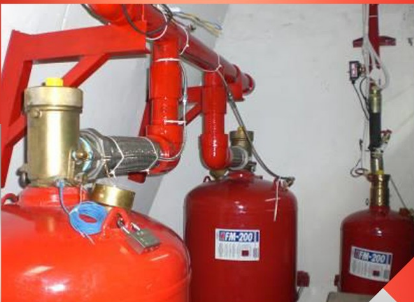
Fire Alarm & Suppression System
