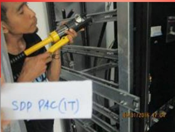
SDP PAC Installation
